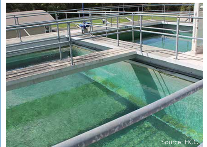
Wastewater treatment plant, Hamilton
