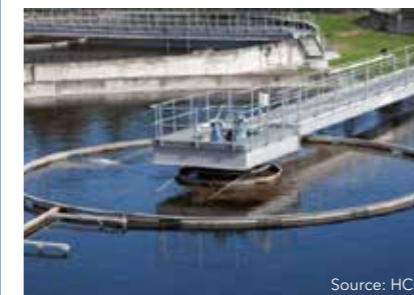
Wastewater treatment plant, Hamilton
